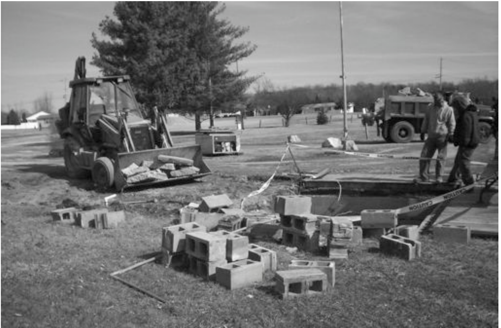
Work has started on the replacement of the marina building. The old building had seen many band-aid repairs over its lifetime including floor rebuild in 2008. The new structure will be an ADA(Americans with Disabilities Act) accessible building measuring 12ft by 34ft with a storage area included. This new building will be a welcomed improvement to the Marina area. Also it is hoped that over the next few years money will become available to upgrade the marina restrooms to meet ADA standards.
